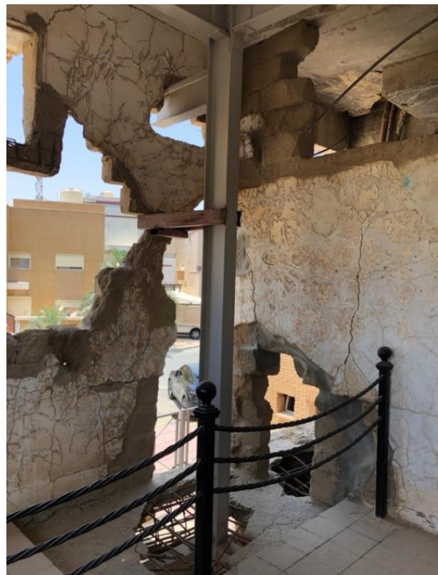
Figure 1. Added barriers for visitor safety (Source: the author 2021)
